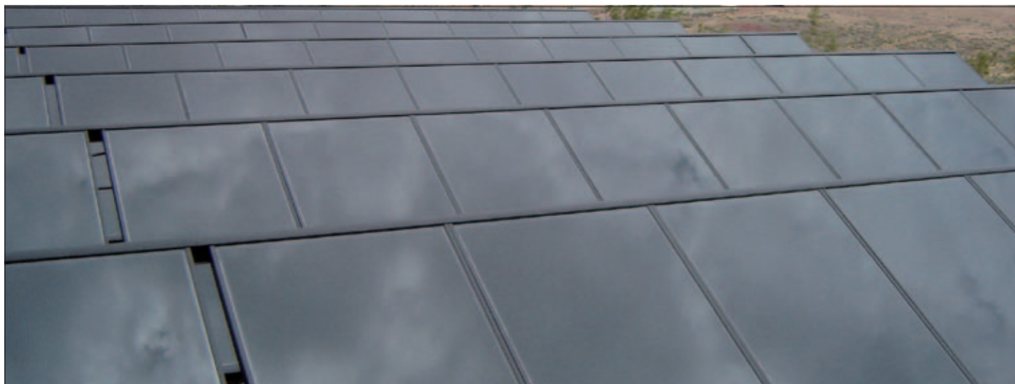
Best quality – higher energy efficiency: Thin-film solar modules in use
